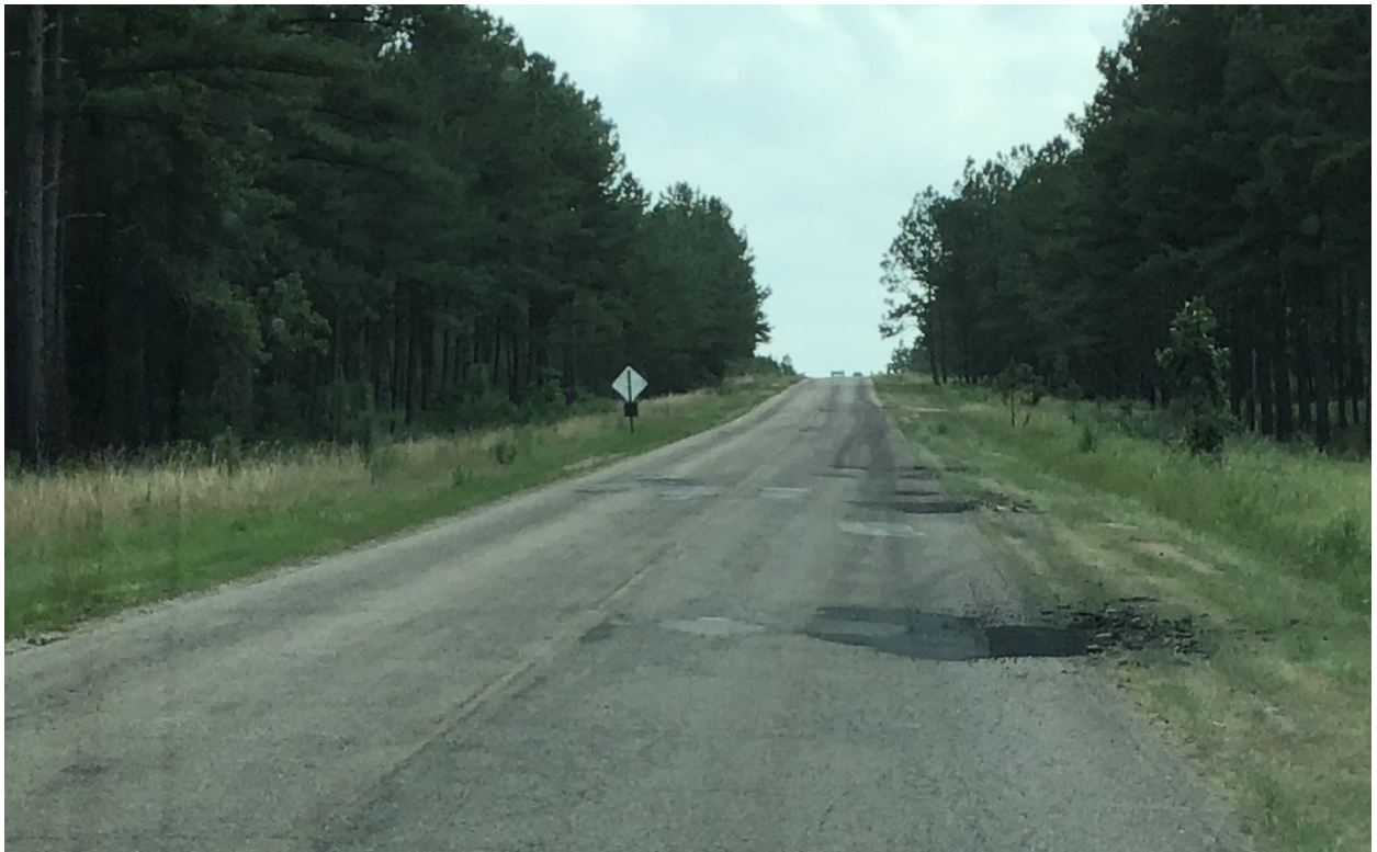
Pavement deterioration on King Road. Striping also needed.
